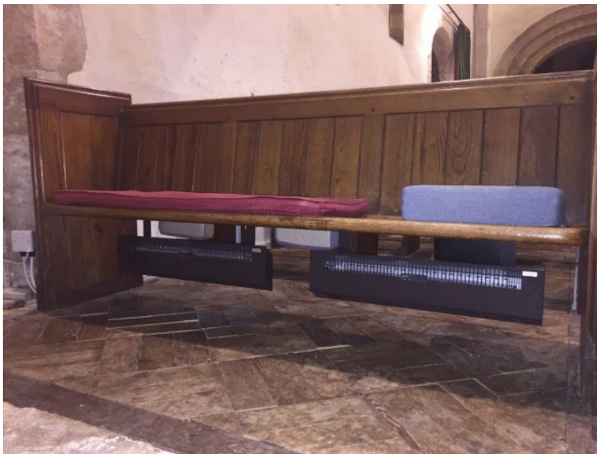
Brown BN Thermic 650W under pew heaters fixed to underside of pew seats for pews which have no solid backs.
